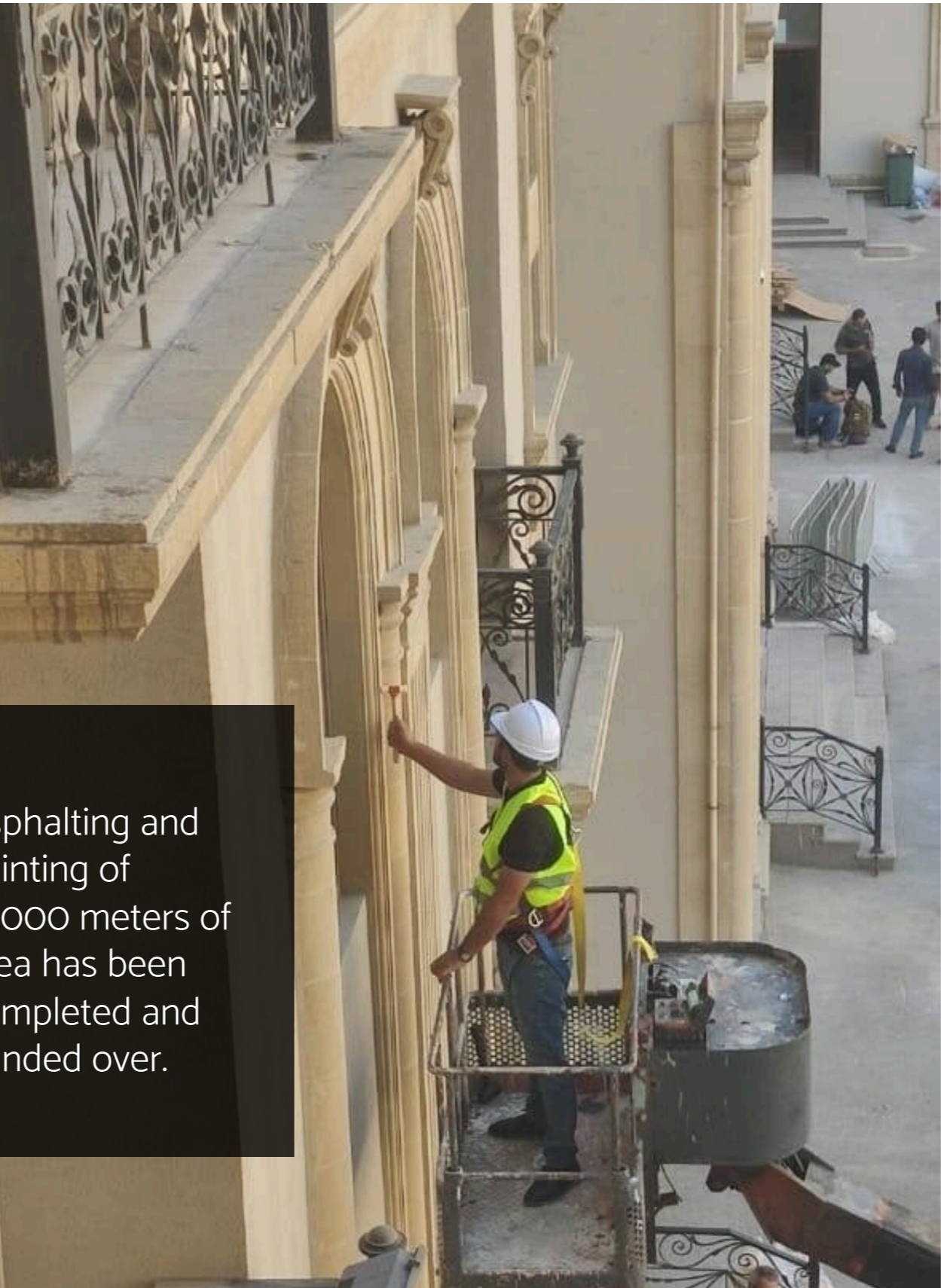
Among the works carried out within the project, facade painting and renovation works were carried out in 11 buildings.
